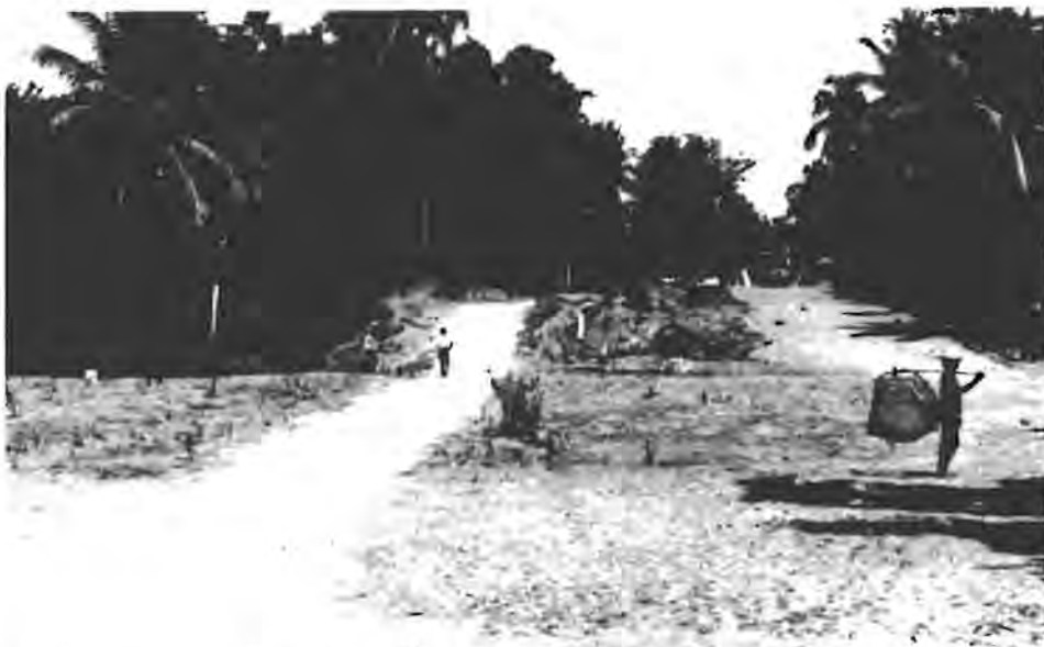
This is one of Mr. Napenias' project--the construction of a feeder road in
